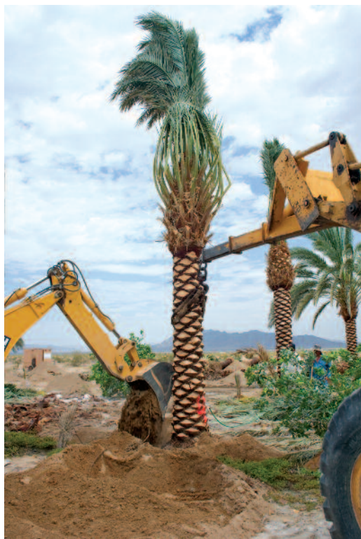
1. The palms were planted and backfilled with the naturally sandy soil at the site (D.R. Hodel).
