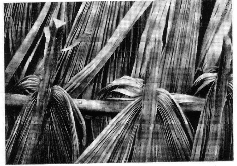
8. Detail showing the manner in which the leaves of Sabal are attached in thatching a roof.
